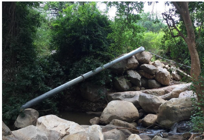
Plate 16.10: Destroyed Section of GI Pipeline
